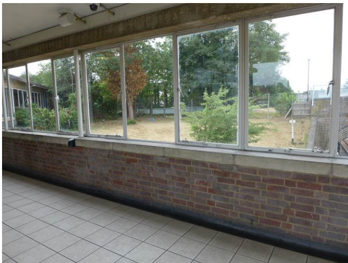
View looking South from Overbridge at approx. position of new lift to serve Platform 1.
